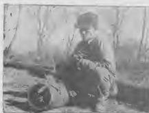
The broken pipe is examined by the foreman. The pilot can locate costly breaks so quickly that the pipeline is fixed in less than half the time usually required.
